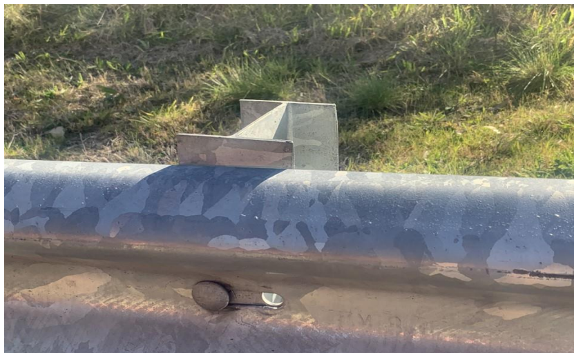
Figure 5: Incorrect installation of safety barrier at Hunter Valley Bus Crash site
